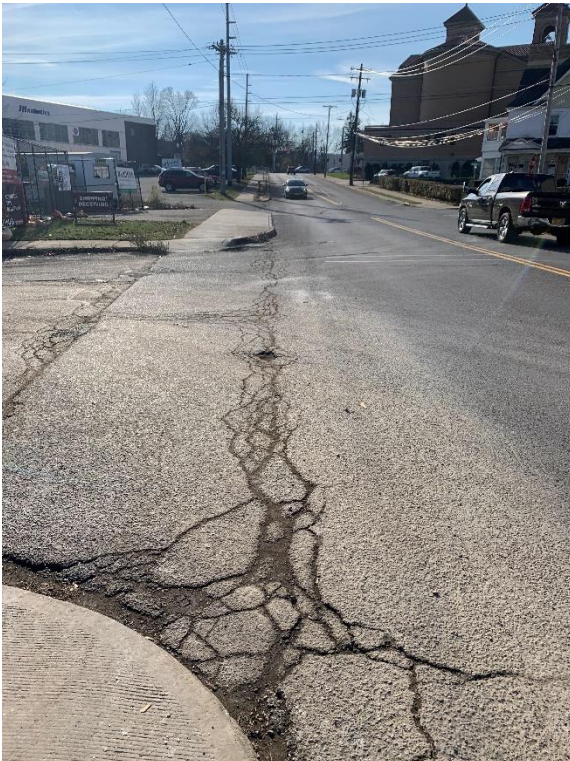
Lack of ADA compliance along westside of Lester Avenue
