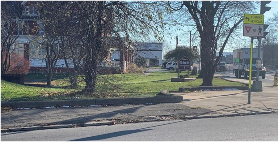
Sidewalk and Curb Conditions west side Lester Ave at Main St
