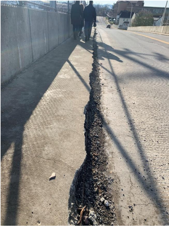
Narrow Sidewalk and Missing Curb on Lester Ave bridge
