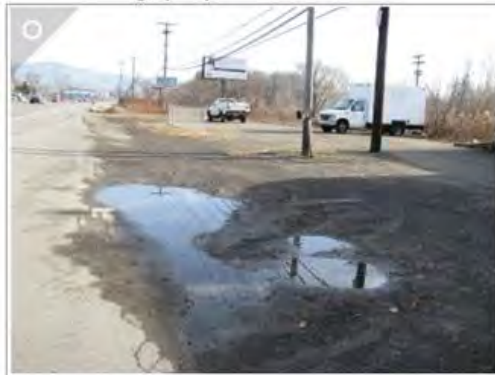
Commercial property with open access to street, no curbs and no drainage facilities. No maintenance required but lack of drainage system contributes to flooding.
