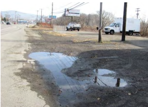
Image 3.3: Lack of stormwater management along Route 11.
