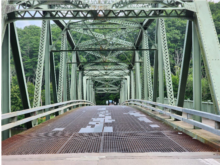
The old steel deck bridge near Chenango Forks on August 3, 2023. (Photo: Bob Joseph/WNBF News)
