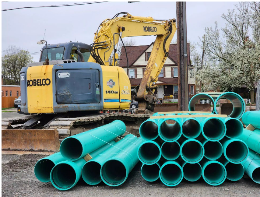
Construction equipment and material staged on the south end of Washington Avenue in Endicott. (Photo: Bob Joseph/WNBF News)
