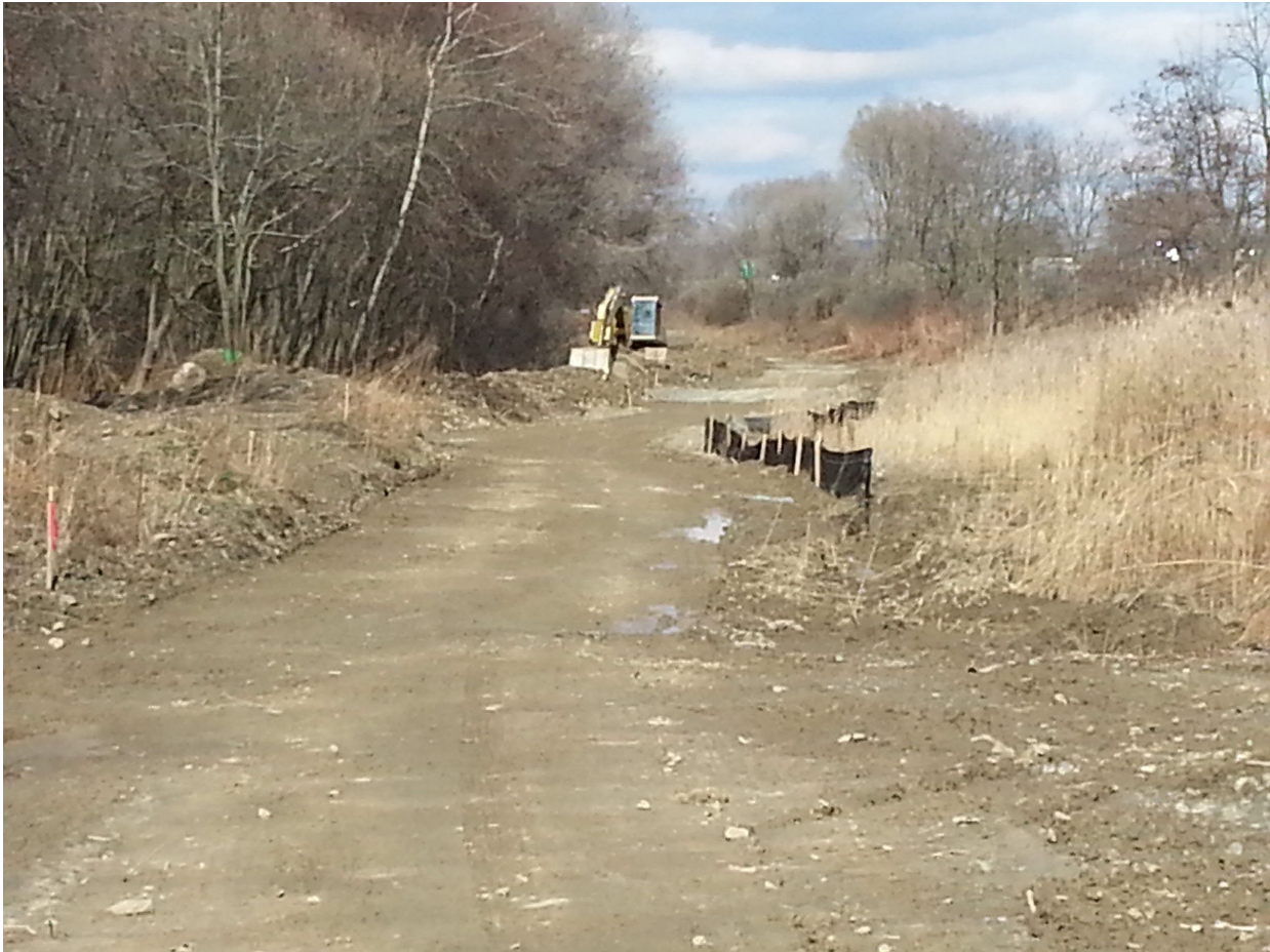
FLASHBACK: A section of the Vestal Rail Trail West under construction on April 14, 2013. (Photo: Bob Joseph/WNBF News)
