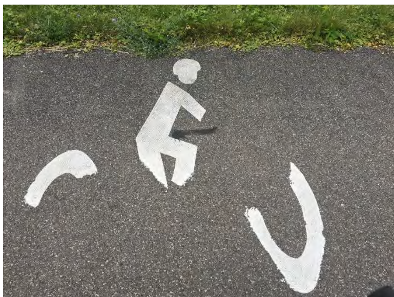
Figure 43 Worn Bike Path Marking
