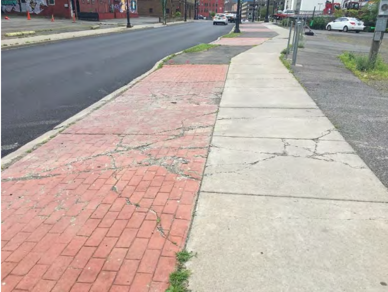
Figure 41 Cracked Cement Next to Driveways
