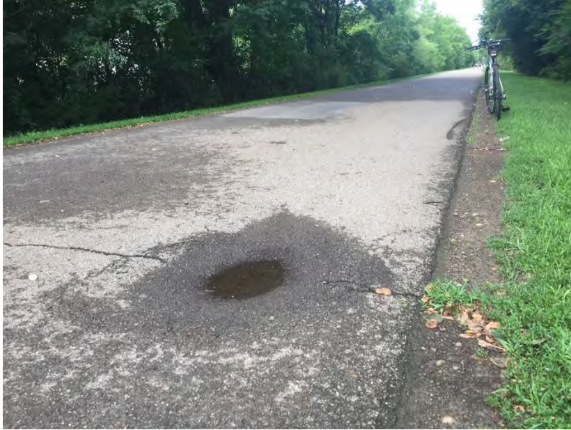
Figure 53 Puddling in Dip in Pavement
