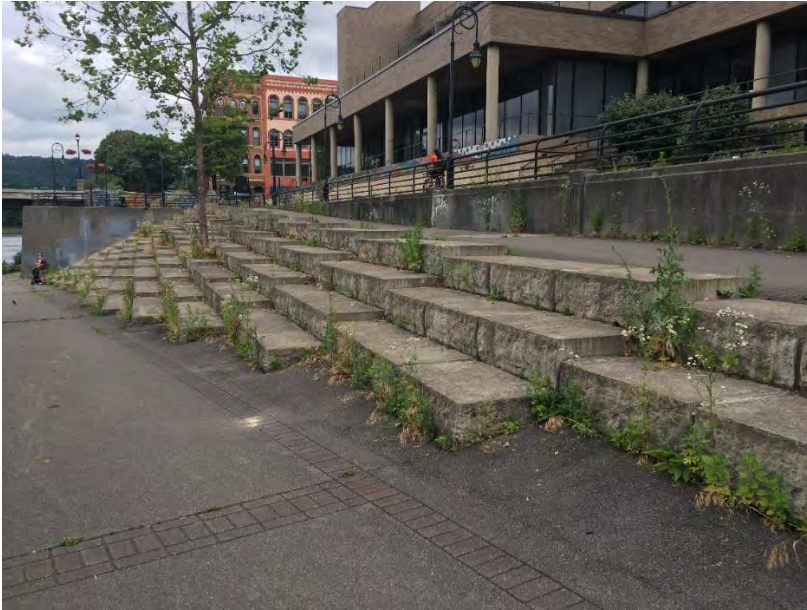
Figure 28 Weeds in Stairs/Seating Area
