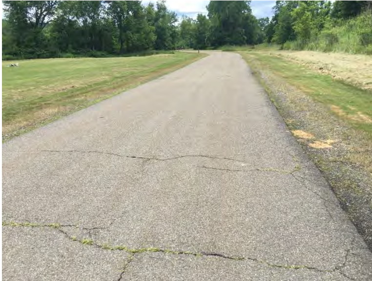
Figure 51 Semi-regular Cracks Across Pavement
