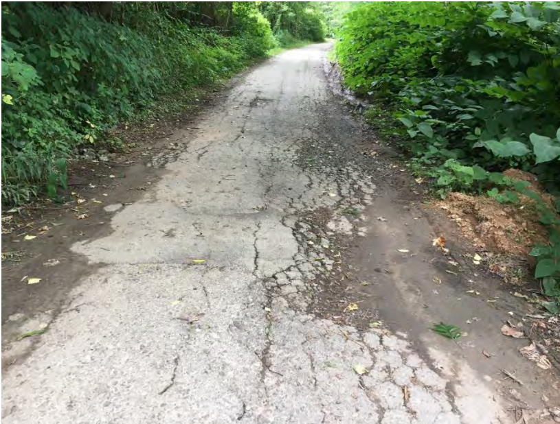
Figure 63 Severe Edge Cracking
