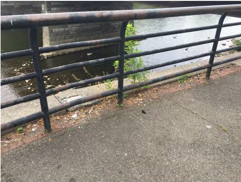
Figure 33 Rust on Railings and Cigarette Butts Along the Edge
