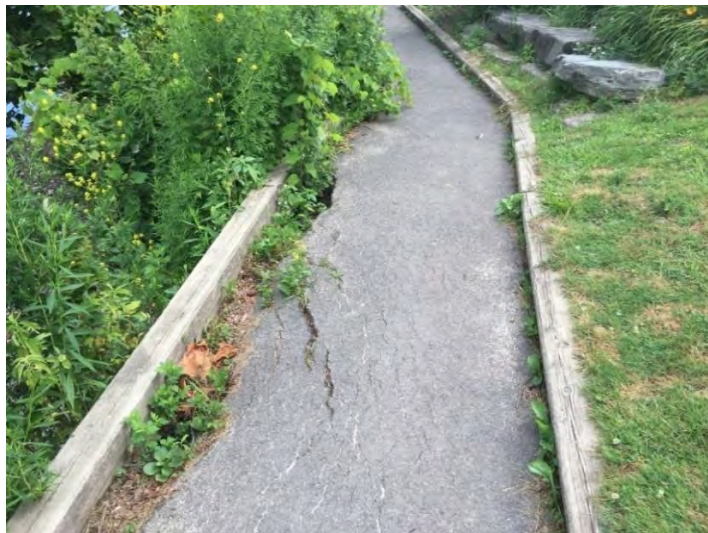
Figure 14 Hole in Paved Bike Walkway
