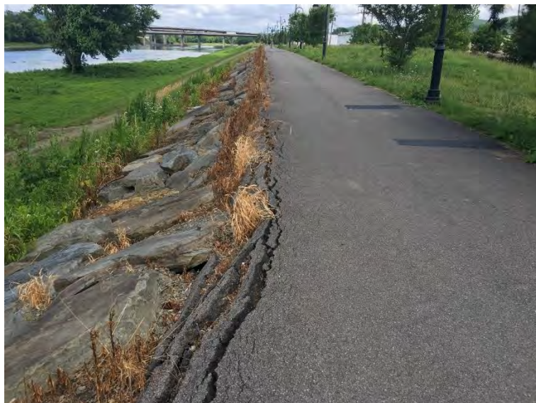
Figure 42 Severe Pavement Cracks at Trail Edge
