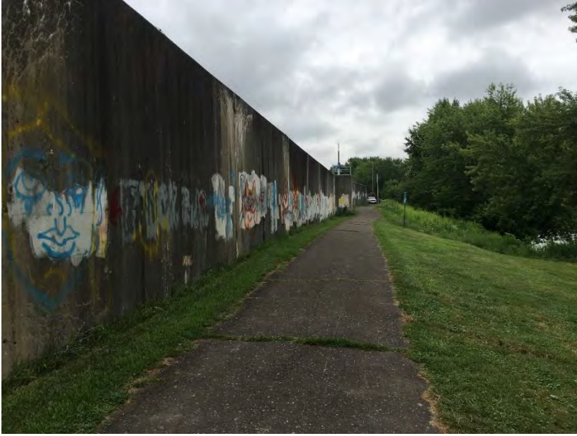
Figure 62 Graffiti Along the Floodwall
