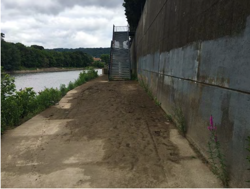
Figure 30 Mud Around Stairwell
