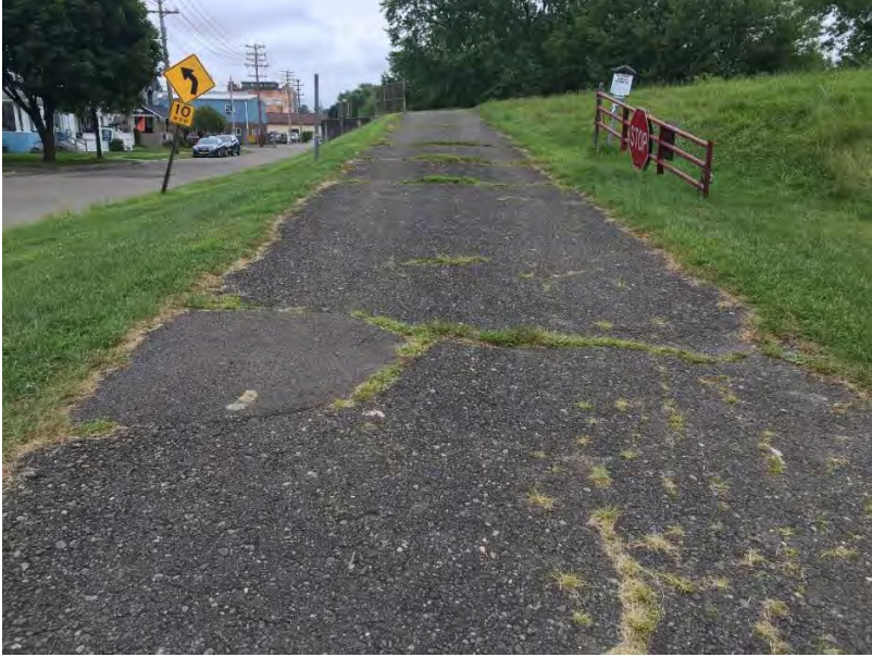
Figure 60 Cracked and Patchy Pavement
