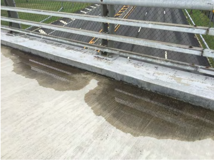
Figure 3 Examples of Puddling on Pennsylvania Avenue Bridge
