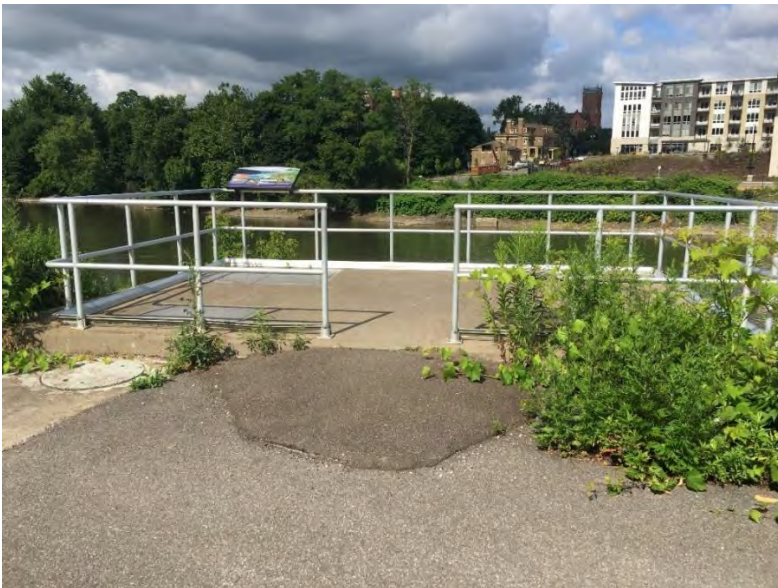
Figure 26 Abrupt Asphalt Ramp to Outlook Platform
