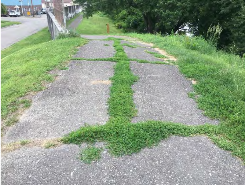
Figure 61 Plant Growth in Pavement Cracks
