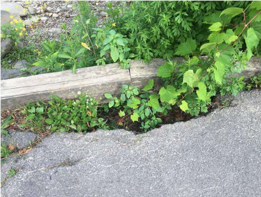
Figure 15 Hole in Paved Bike Walkway Close-up
