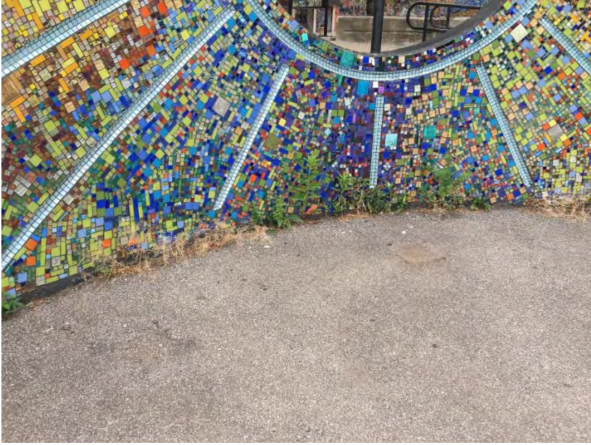
Figure 34 Wear, Rust, and Weeds in Mosaic Area
