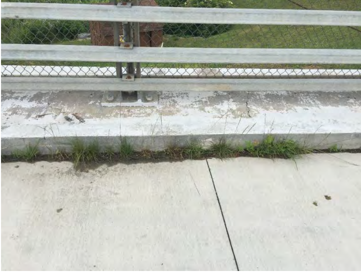
Figure 5 Weeds and Dead Grass Residue Along Cement Trail Portion
