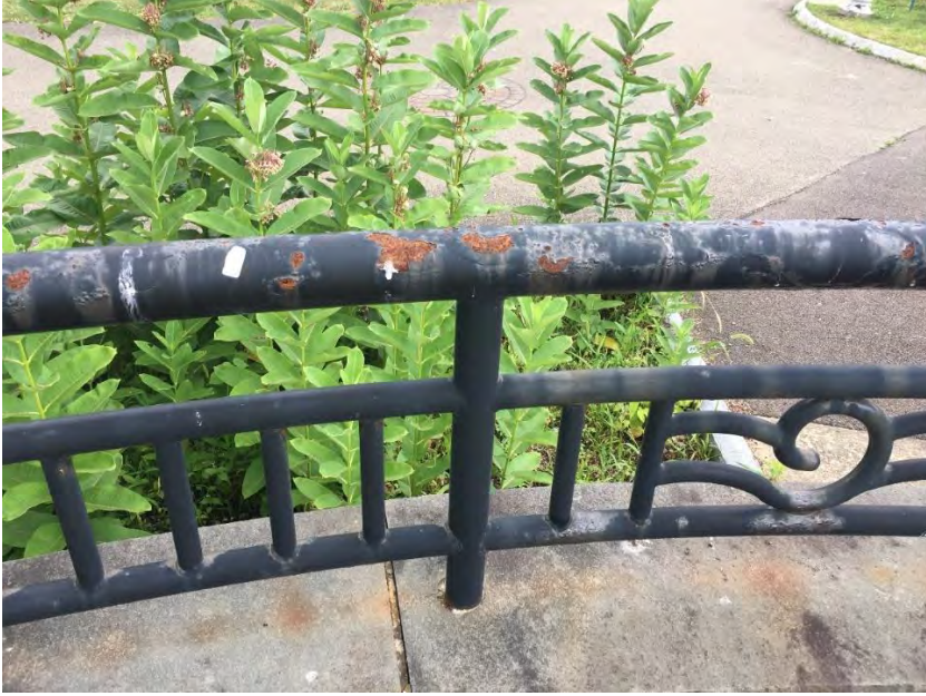
Figure 17 Chipped Paint and Rust
