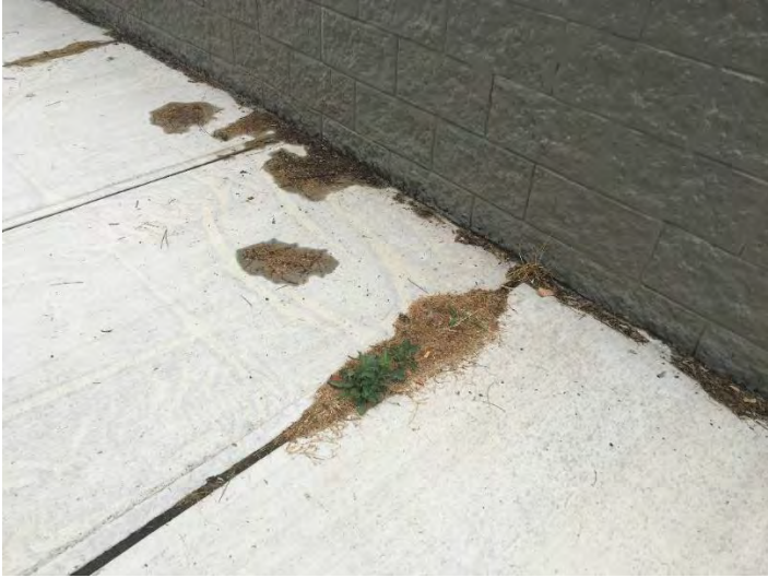
Figure 4 Dead Grass Residue Along Cement Trail Portion
