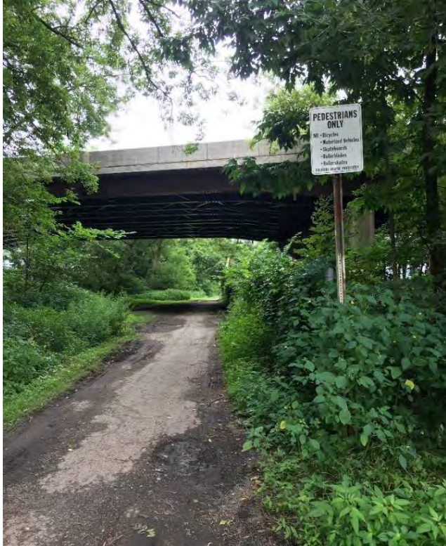
Figure 64 Cracked Pavement Especially Along the Side
