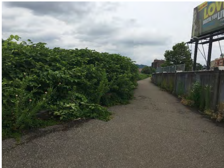
Figure 22 Severely Overgrown Vegetation and Weeds on the Side of the Floodwall
