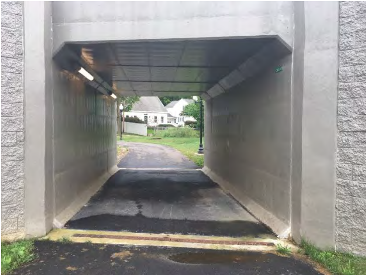
Figure 6 Puddling Near Tunnel
