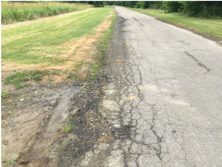
Figure 50 Cracks on Side of Pavement
