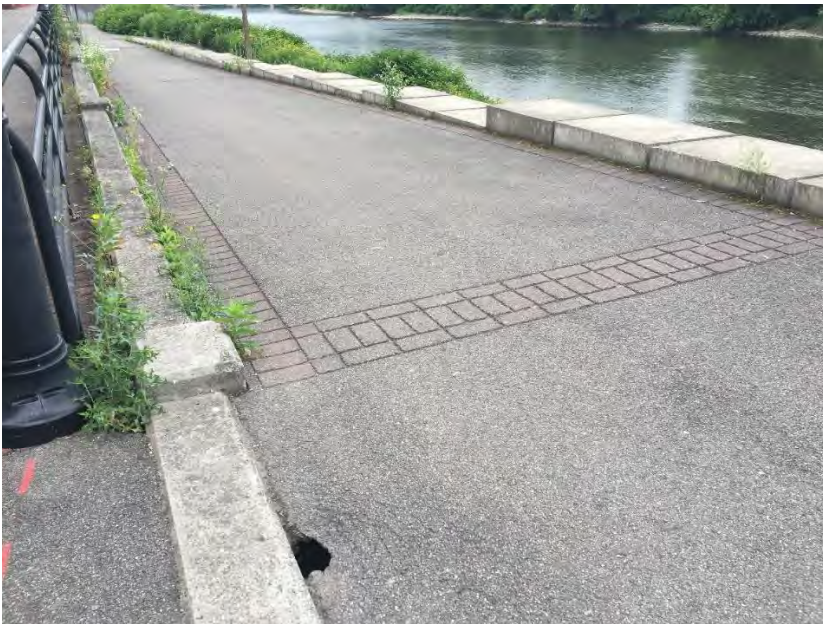
Figure 31 Deep Hole in Pavement Near Traffic Counter
