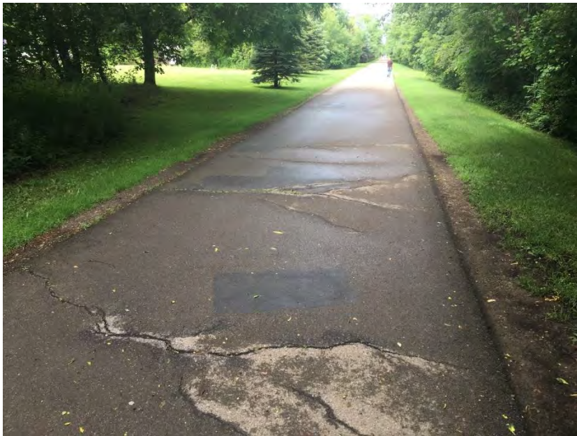
Figure 54 Significant Bumps and Cracks
