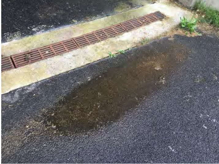
Figure 7 Puddling Near Tunnel Close-Up
