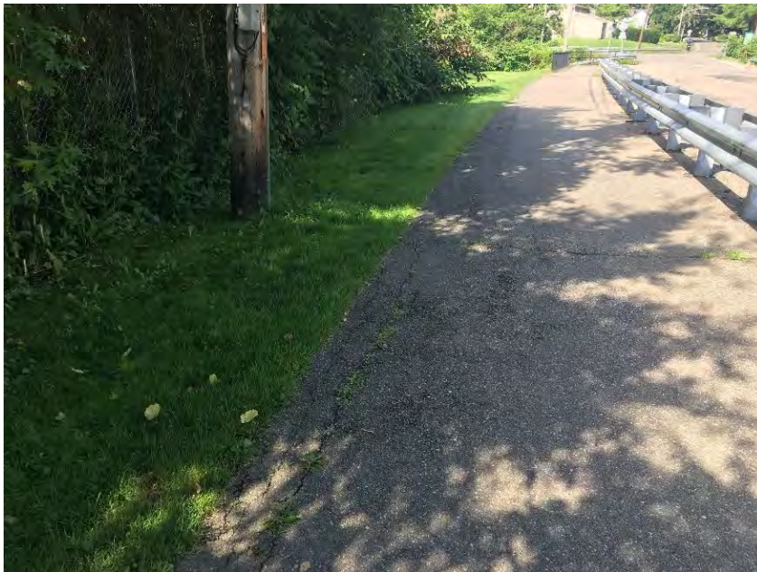
Figure 56 Slight Cracks in Pavement
