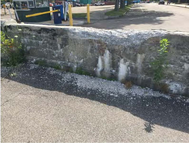
Figure 25 Rock Debris from Floodwall Adjacent to Outlook Platform
